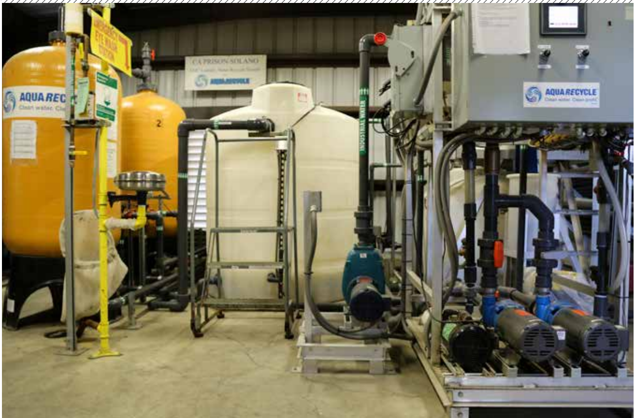
CALPIA operates new laundry reclamation systems
