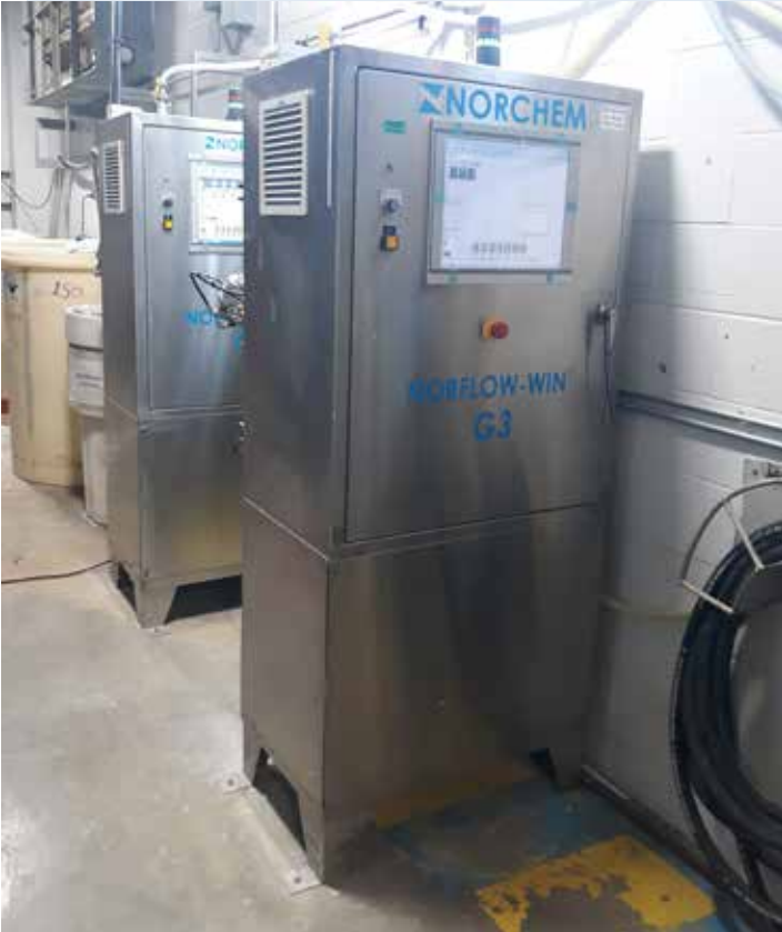
CALPIA's new laundry automation equipment reduces water, energy and chemical usage
