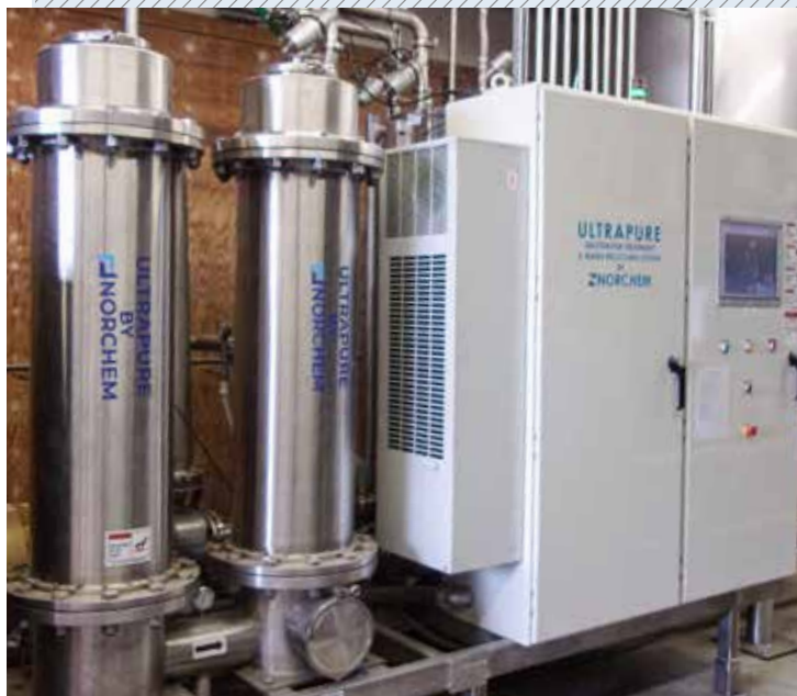
CALPIA's laundry automation equipment at the California State Prison, Los Angeles County
